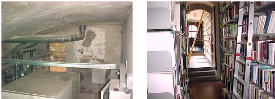
Figure 8: Heating plant and part of interior.
